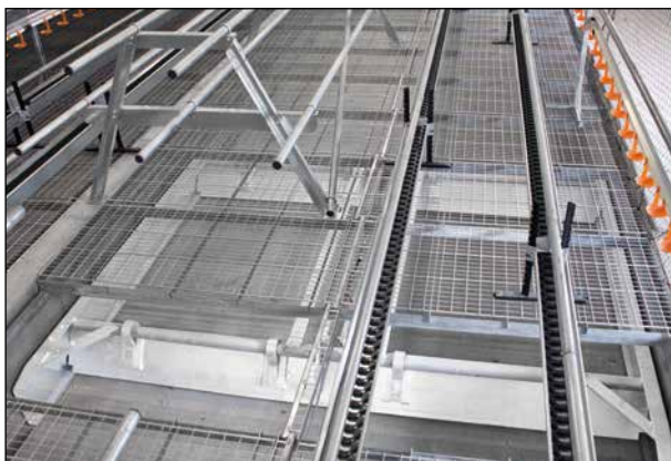
▲ Dung flap scraper below rust
