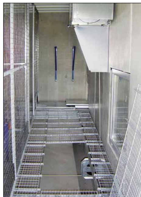
▲ Staff passage with inspection door
