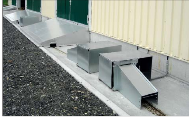
▲ Drive winches EW4 and cross canal covering
